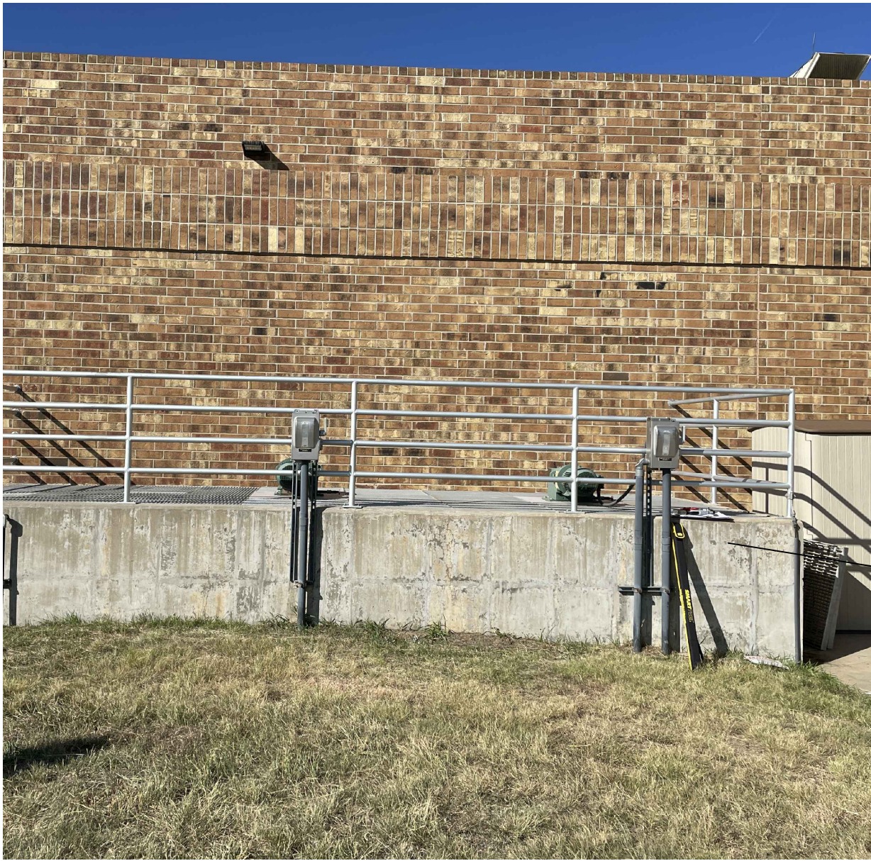
EXISTING RAPID MIXING BASIN
