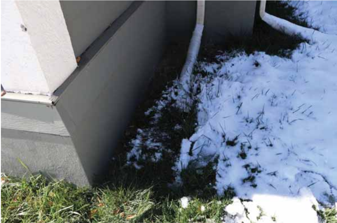
Image 24: Drainage System, Gutters & Downspouts_ Discharge is too close to the foundation
