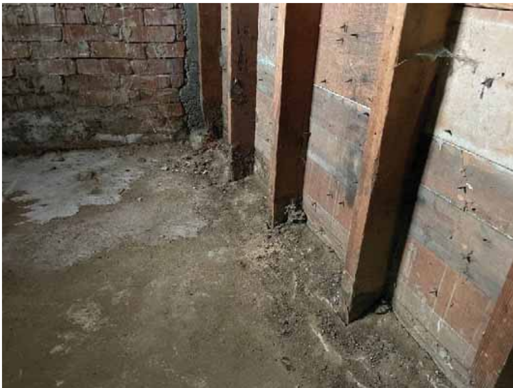
Figure 16: Deteriorated studs in basement Room-4
