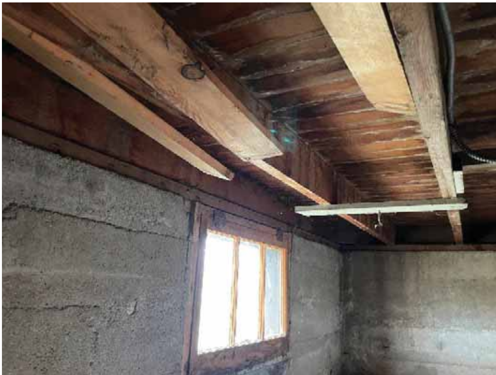
Figure 10: Water staining at porch framing
