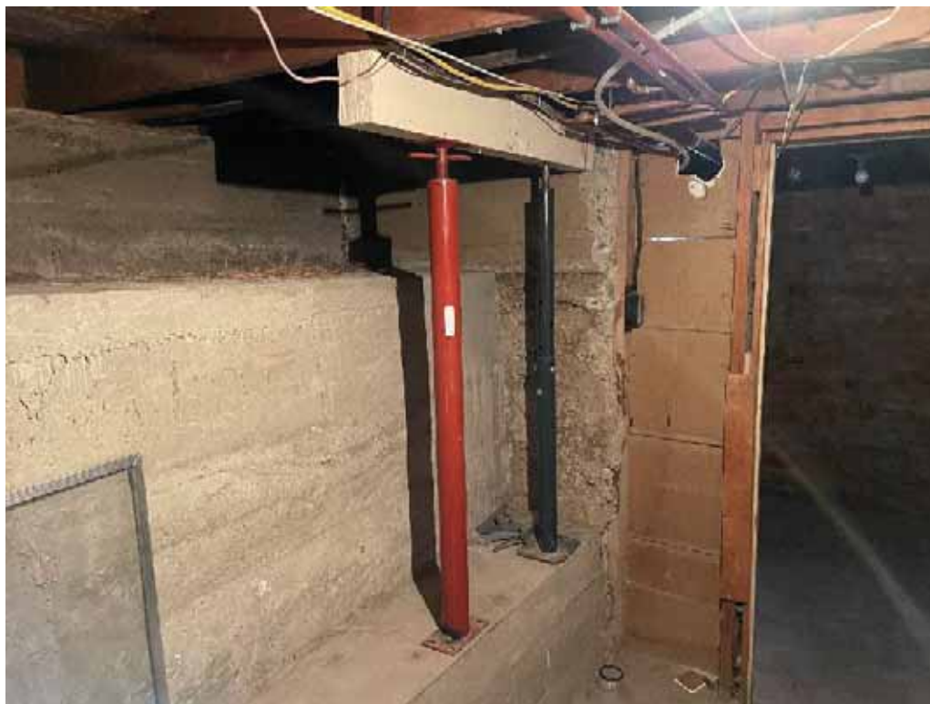
Figure 12: 4x6 dropped beam on jack posts in basement Room-9. Note that posts are not anchored, just friction-fit
