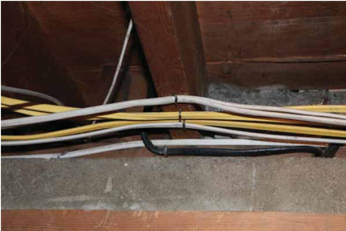
Image 41: Electrical Distribution System_ Wiring improperly attached to exposed edge of joists
