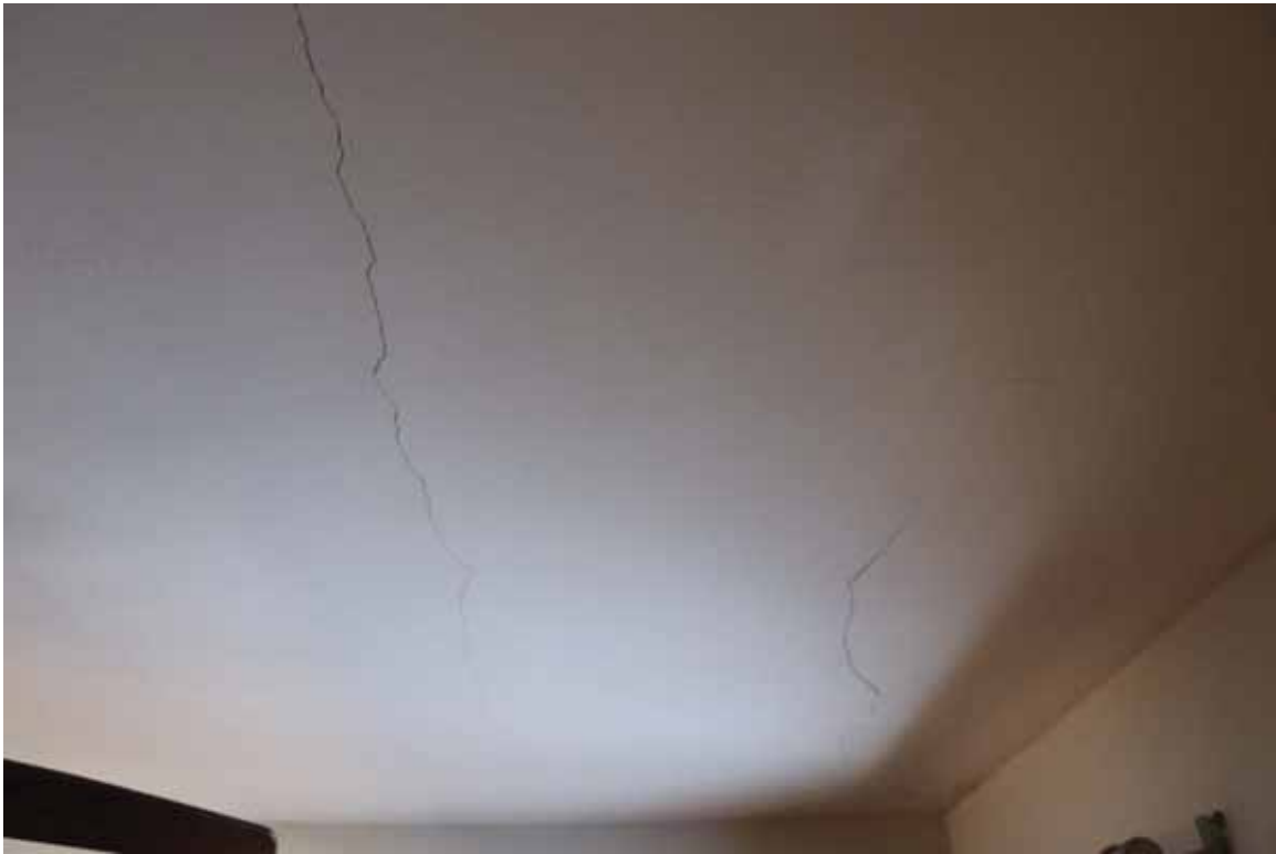
Image 32: Ceiling Finish Materials_ Ceiling cracks in bedroom
