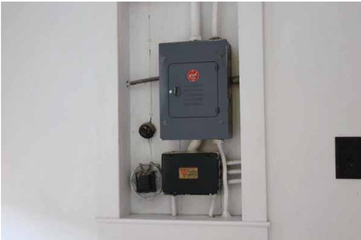
Image 40: Electrical Service & Panels_ Federal "NoArk" panel and unknown associated electrical devices
