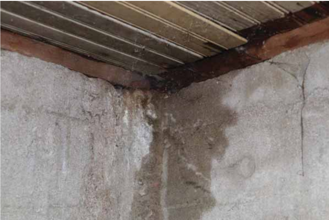
Image 25: Drainage System, Gutters & Downspouts_ Active water infiltration in basement directly adjacent to previous photo of downspout
