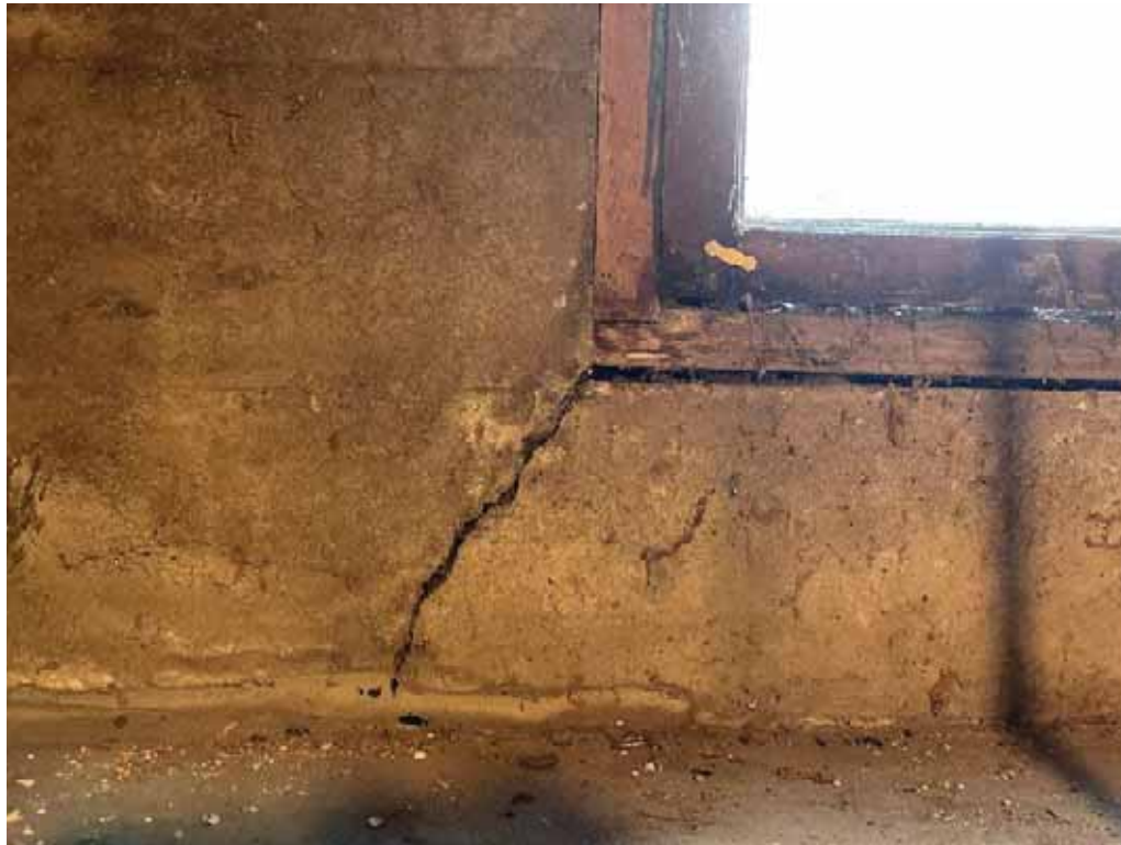
Figure 5: Settlement (or shrinkage) crack under window in west basement wall
