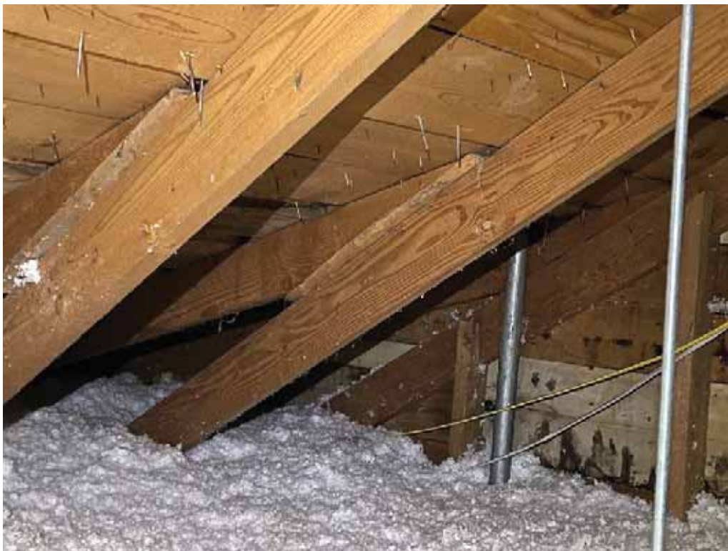
Figure 14: Typical shed rafter to main roof rafter connection. No connectors visible.
