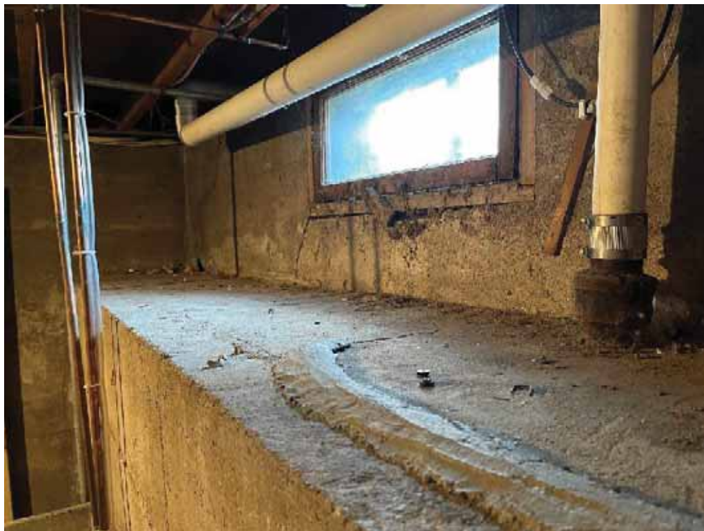
Figure 6: Repaired separation crack between top of retaining wall and concrete cap at west basement wall
