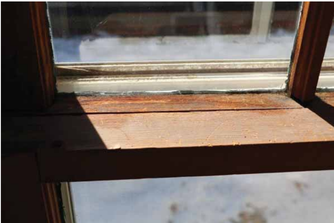
Image 29: Windows_ Typical level of deterioration
