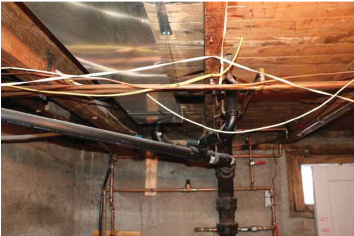
Image 42: Electrical Distribution System_ Wiring improperly attached to exposed edge of joists
