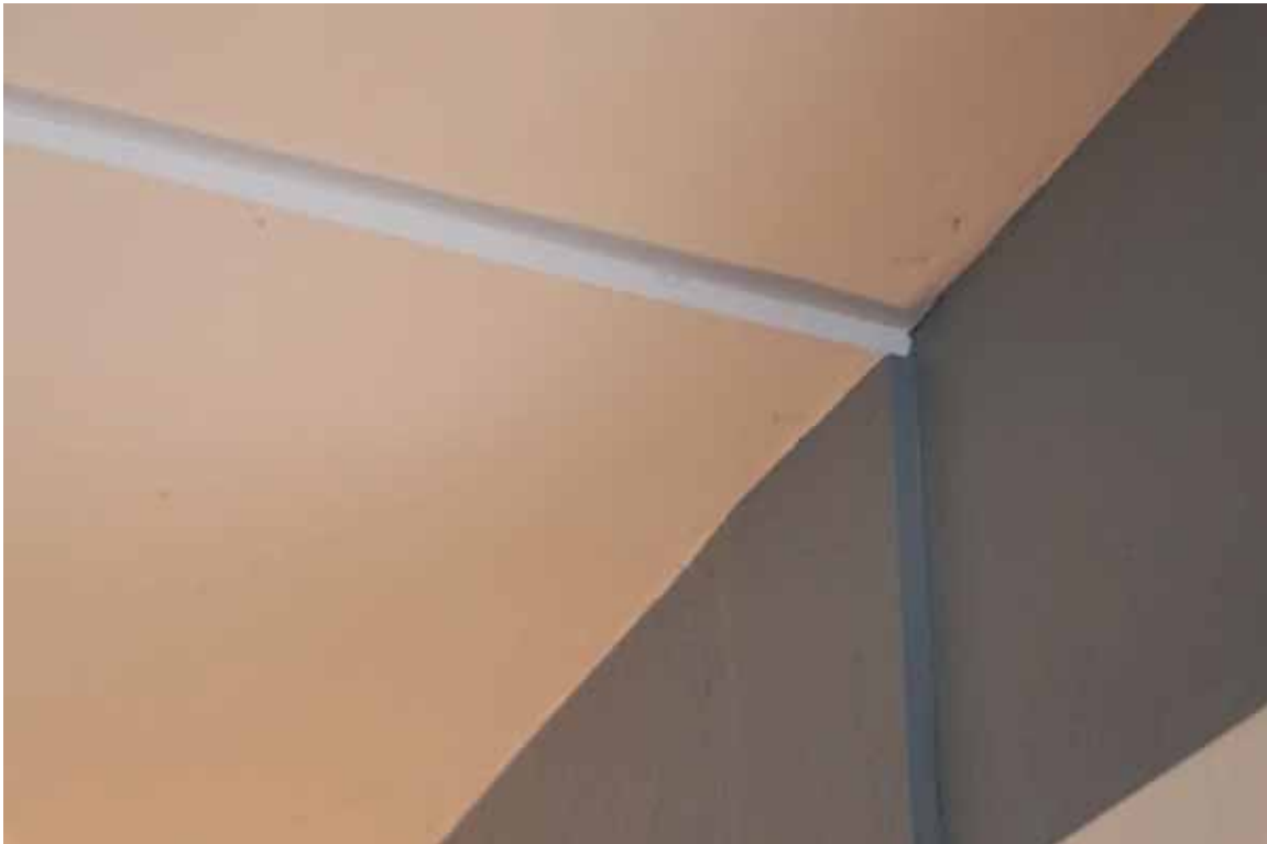
Image 31: Wall Finish Materials_ Drywall/plaster seam at the kitchen
