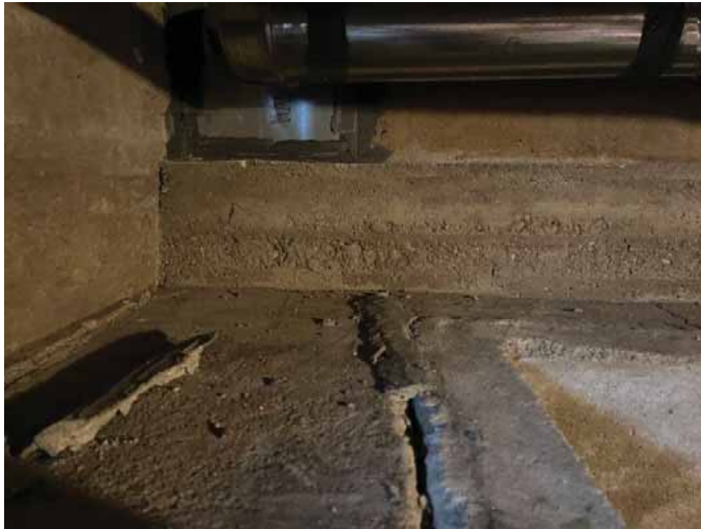
Figure 7: Repaired separation crack between top of retaining wall and concrete cap at west basement wall
