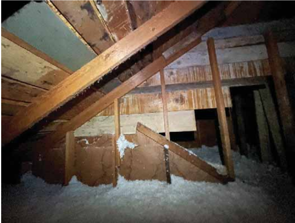
Figure 17: Discontinuous studs in east gable end wall
