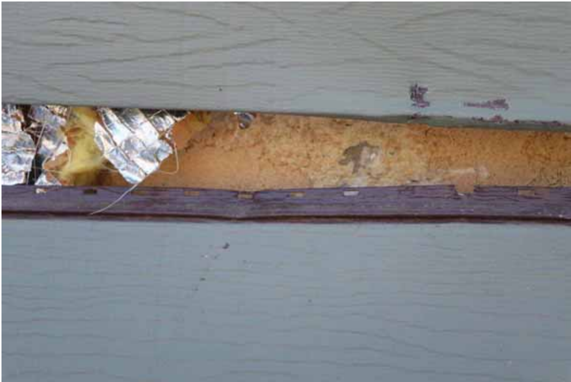
Image 19: Exterior Finishes_ A section where the siding has slipped shows the stucco underneath
