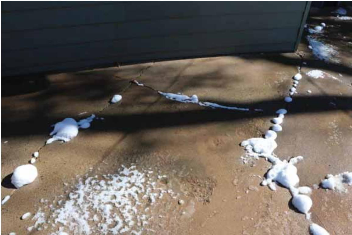
Image 23: Perimeter Foundation Drainage_ Concrete poured up against the rear of the home is cracked and allowing surface water in penetrate
