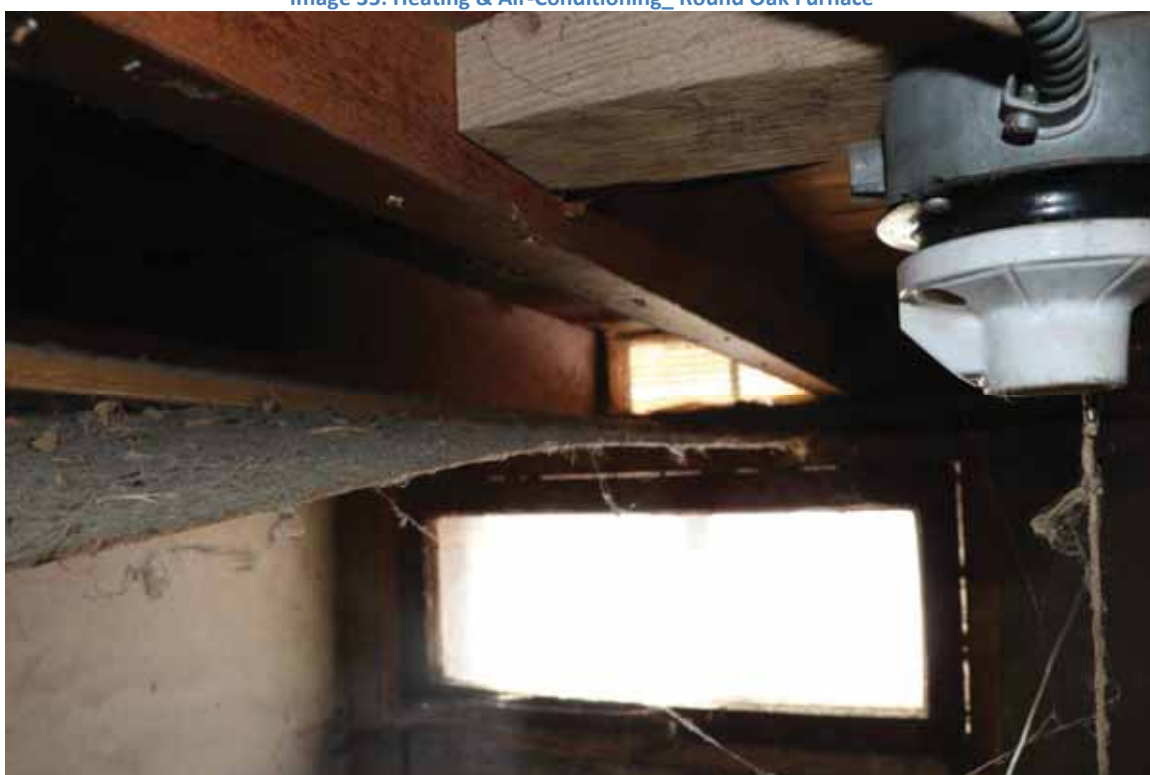
Image 36: Heating & Air-Conditioning_ Supply air duct for furnace has failed
