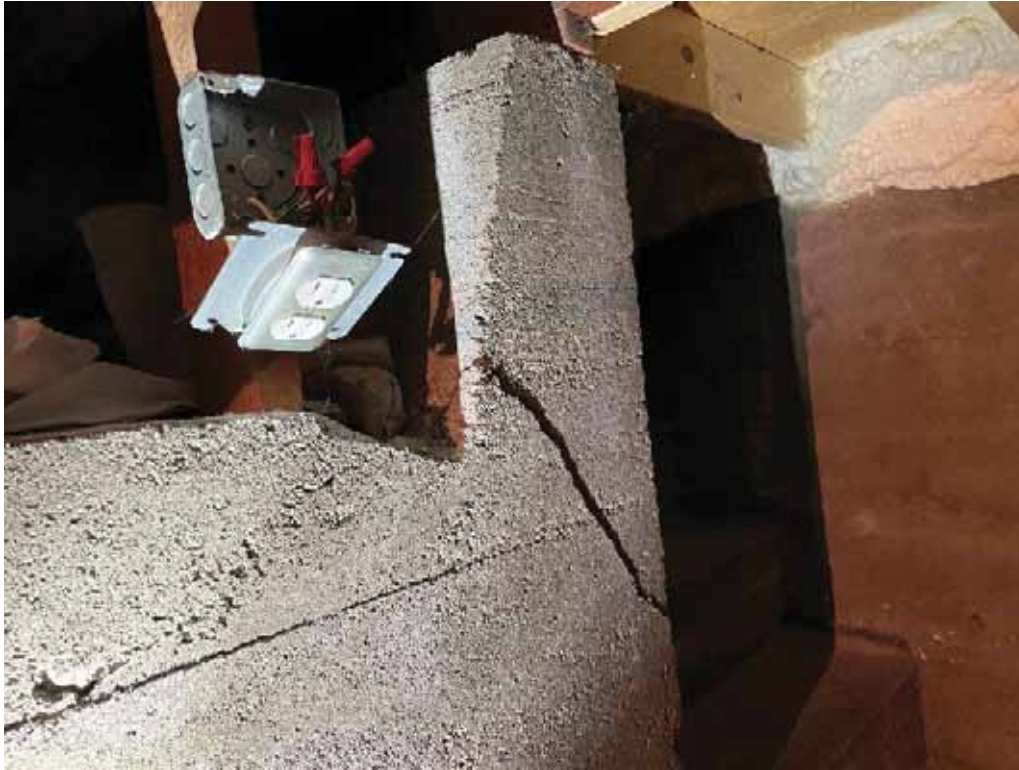
Figure 9: Presumed settlement crack at unused basement stair west side
