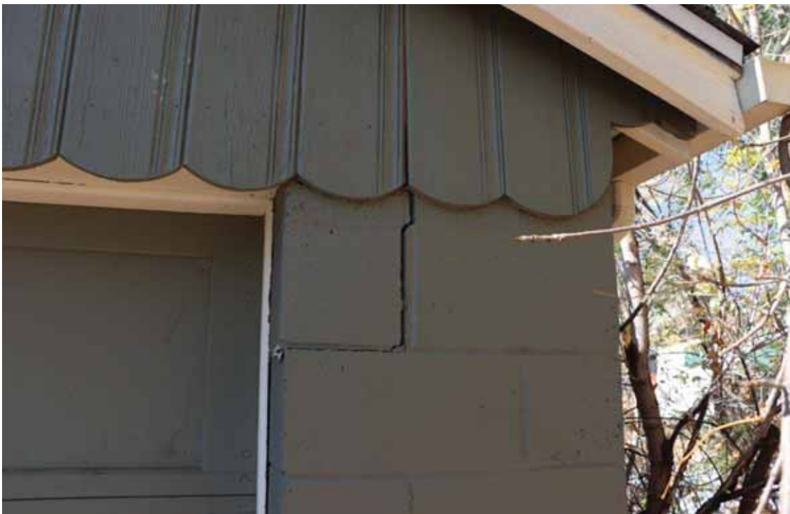
Image 6: Associated Landscape Feature Detached Garage Crack by door
