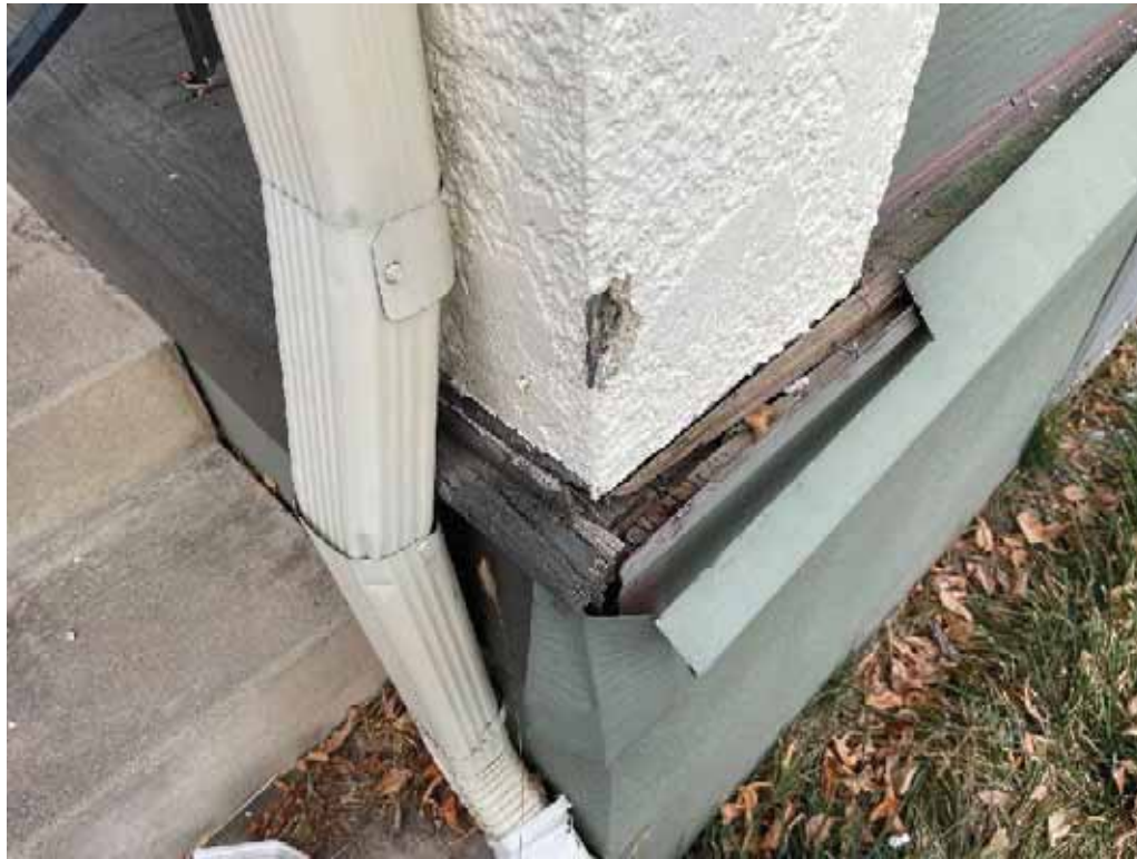
Figure 11: Deterioration at southeast corner of porch
