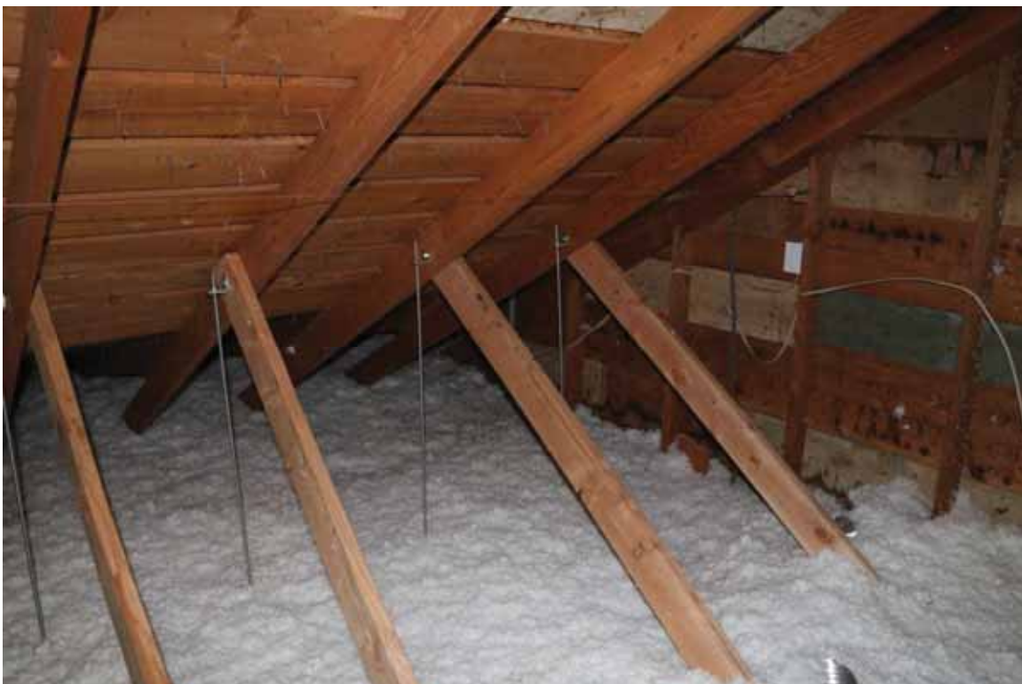
Image 15: Roof Framing Systems_ Note the vertical metal tie rods. As they are attached with L-brackets, it is assumed that they are not designed to carry much weight
