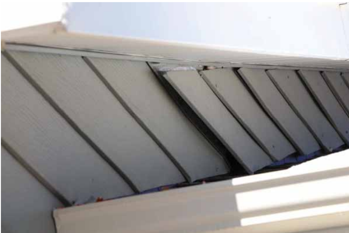
Image 20: Exterior Finishes_ Loose siding
