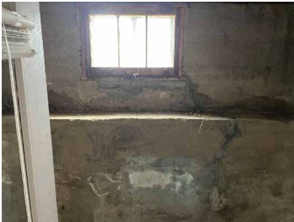
Figure 8: Shrinkage crack in east basement wall under porch
