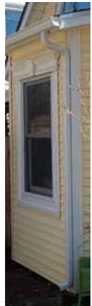
Typical gutter & downspout without an extension
