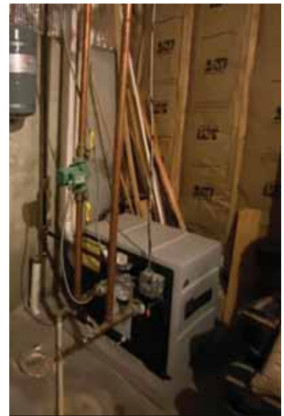
High efficiency boiler
